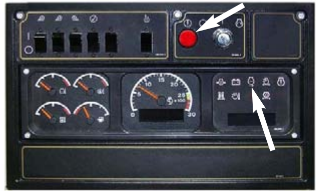
Fig. 113: Coolant Flow Indicator.
