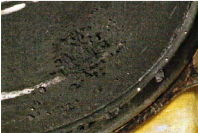
Fig. 48: Effects of improperly treated cooling system.
